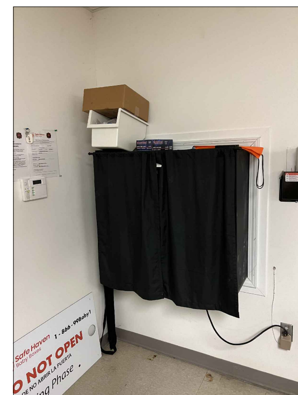
Existing Baby Box interior installation for reference.
