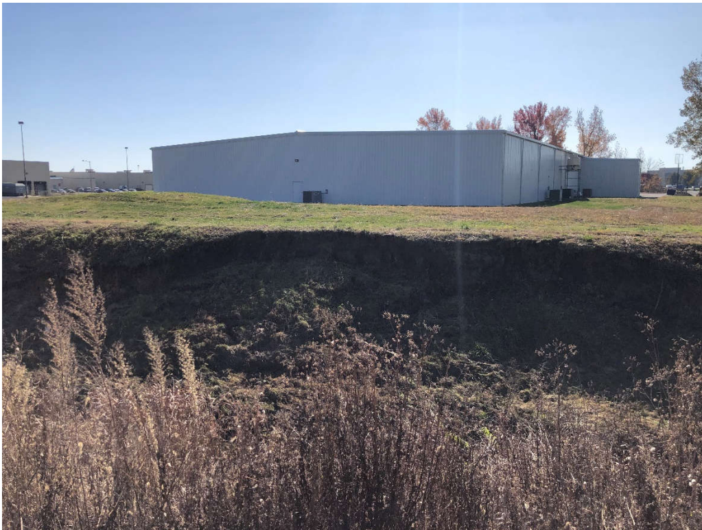
Wabash Erie Canal bank destabilization-Picture from Northern Bank
