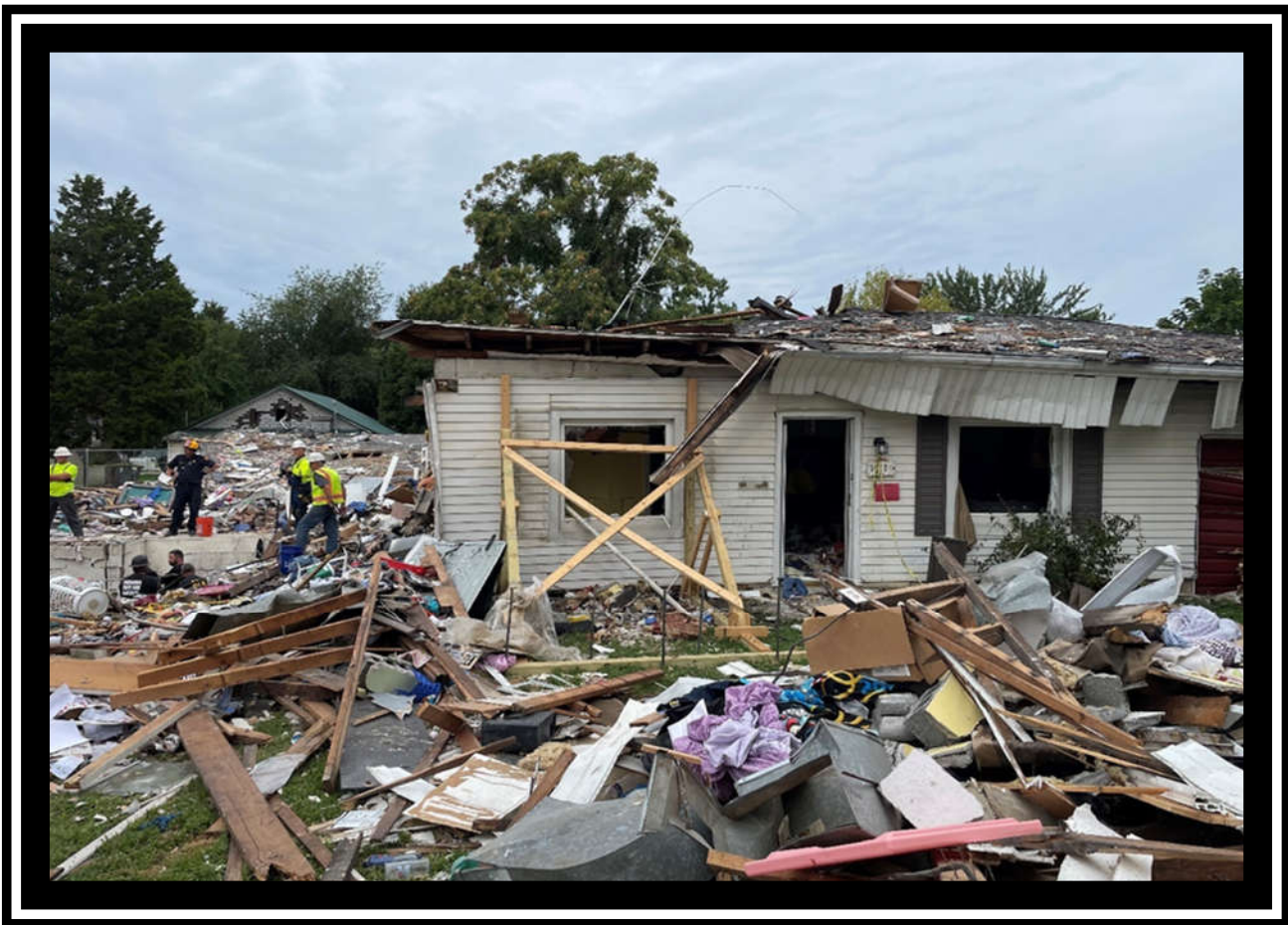
Shoring executed by the TRT to conduct searches after the Weinbach Ave. explosion on August 10, 2022.
