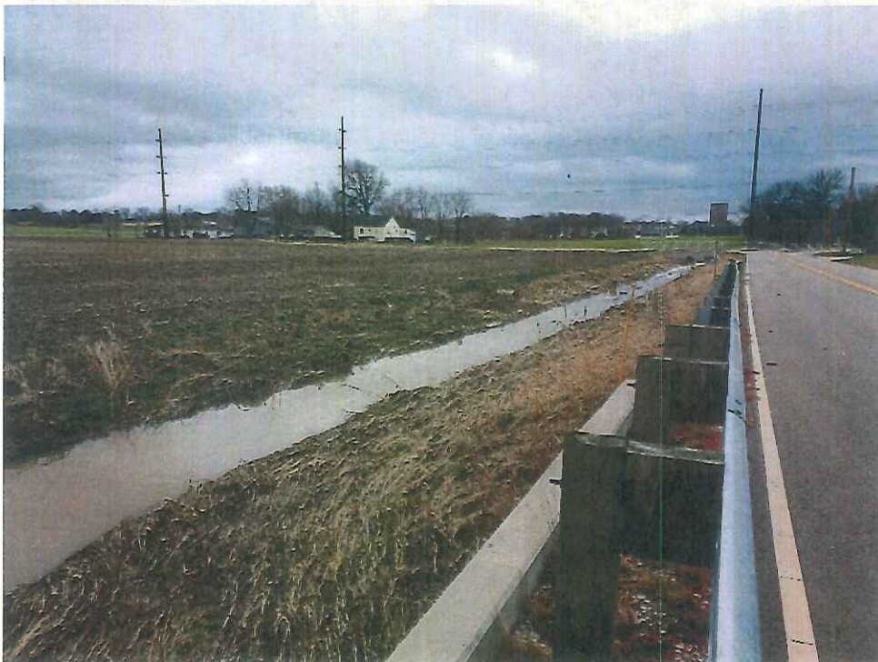
March 7, 2022 - ditch on the east side of Korff Road looking south
