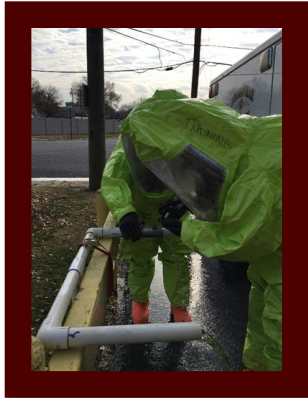
Leak Control in Level A
